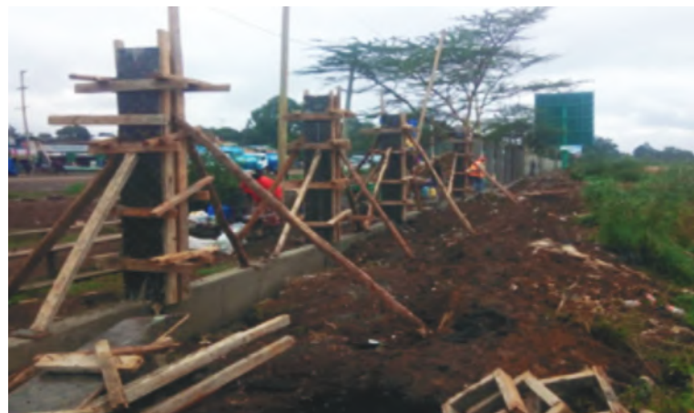
Ongoing construction works of a masonry perimeter wall. The land is at the junction of Langata Road and Ngong Road.
